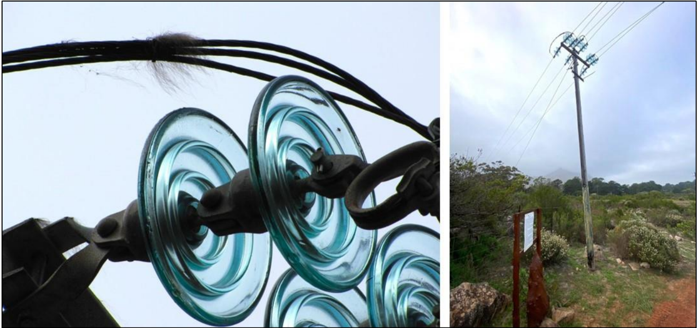
Figure 16. Baboon hair on the live wires of the pole outside Baskloof. The pole was greased by the electricity department within 48 hours of the incident.
