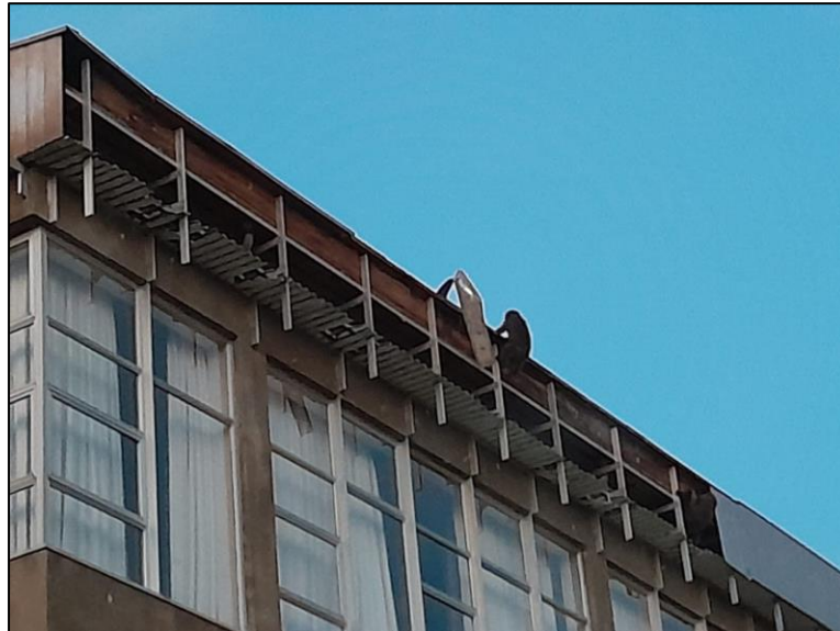
Figure 13. Baboons gaining access through the damaged roof above the galley in Waterfall Barracks.
