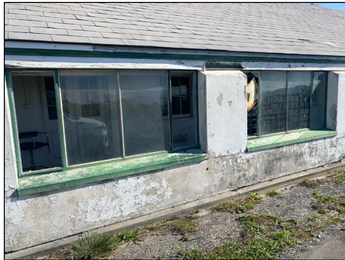
Figure 8. Broken windows at Signal School.
