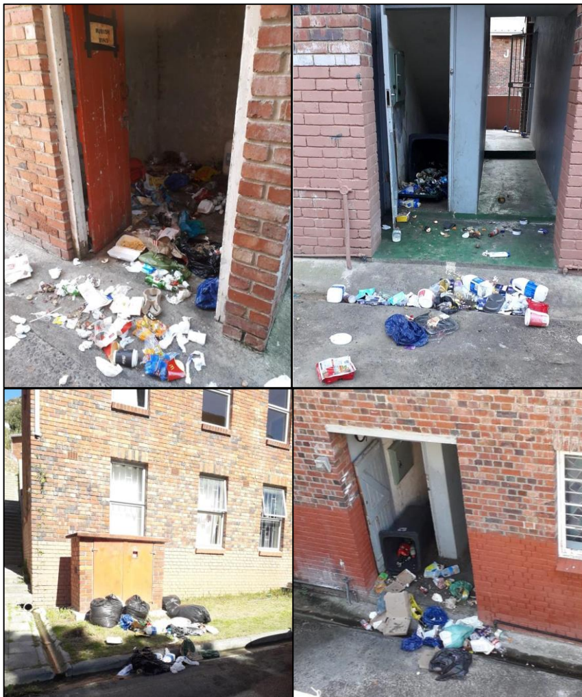
Figure 2. Insufficient waste management and infrastructure maintenance at SA Navy properties.
